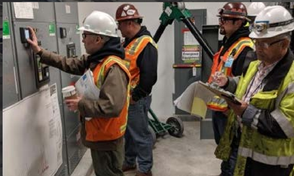
Emergency power trials
